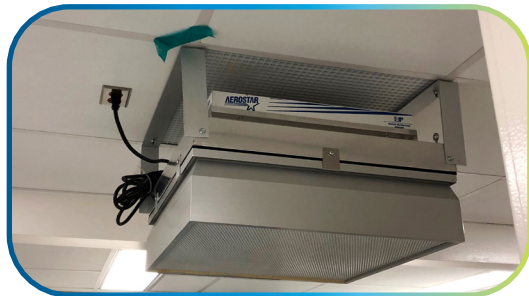
Filtration Unit Installed Below Supply Air Vent
